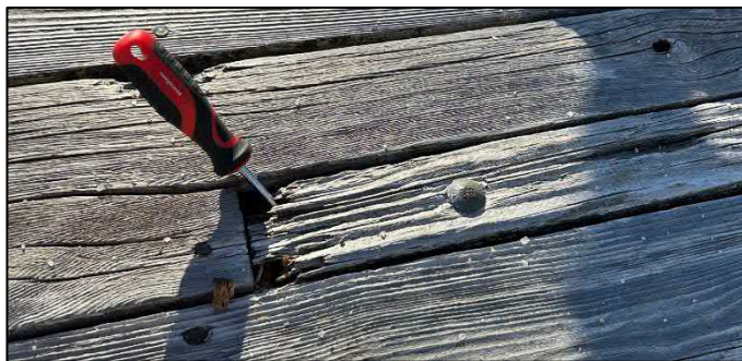
Figure 36 - Example of Decayed Connection Member at Finger Connection to Wing Dock
