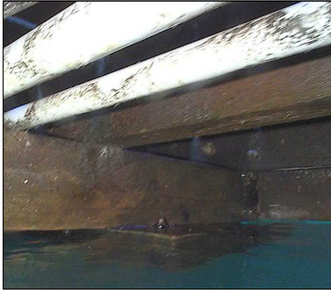
Figure 43 - Sagging Framing Near Slip B7 on Dock B – Near Location of Attached Float
