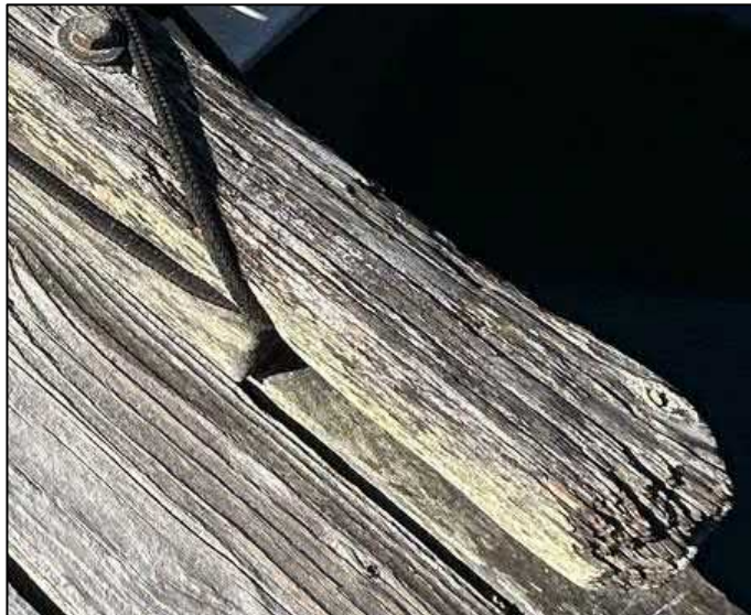
Figure 35 - Example of Decayed Bull Rail
