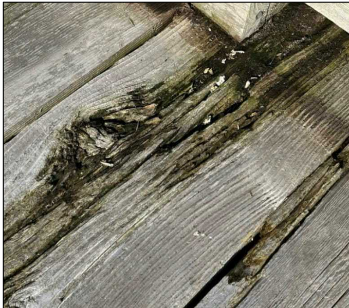
Figure 27 - Example of Deck Board Decay
