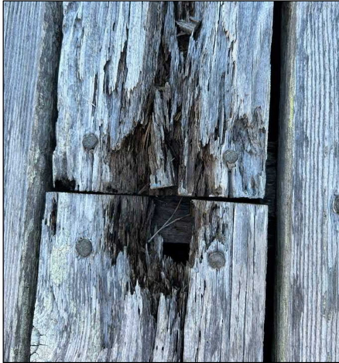
Figure 30 - Example of Deck Board Decay
