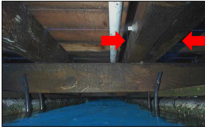
Figure 8 - Typical Configuration - Underside Wing Dock – Showing Spliced Stringer Connection (Spliced connection identified with red arrows.)
