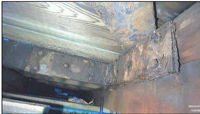
Figure 55 - Example of an Extensively Corroded Connection Plate Between Wing Dock and Main Dock
