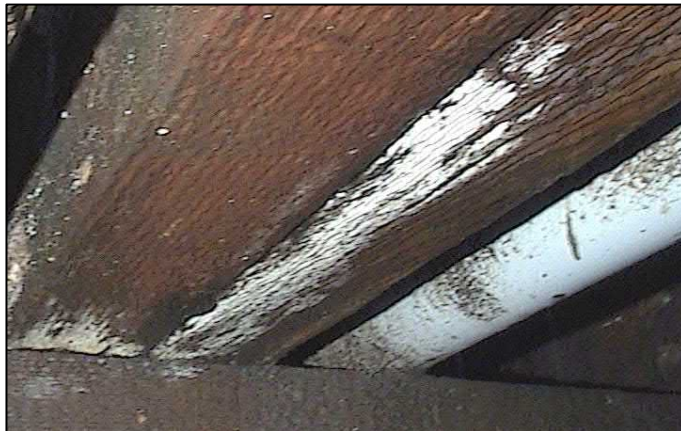
Figure 50 - Example of Fungal Growth on Framing
