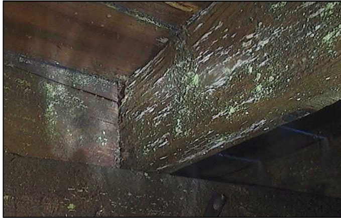
Figure 51 - Example of Fungal Growth on Framing
