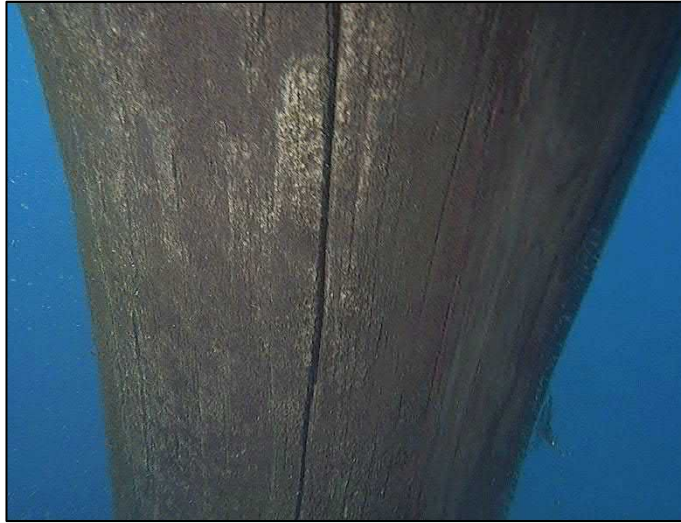
Figure 63 - Typical Crack in Timber Pile
