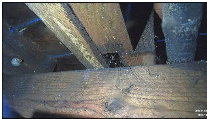
Figure 42 - Disjointed Connection Near Slip B6 on Dock B
