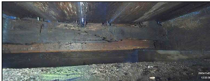
Figure 46 - Decayed Framing on Finger Near Slip C30 on Dock C
