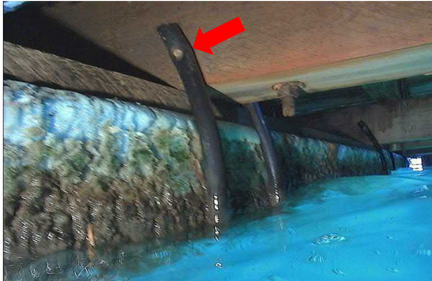
Figure 22 – Typical PVC Connection Straps for Polystyrene Billets (The red arrow identifies the single nail connecting the PVC strap to the timber framing.)
