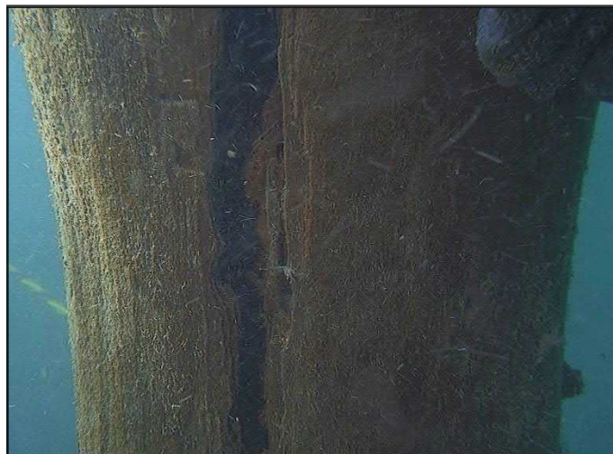
Figure 64 - Typical Decayed Timber Pile
