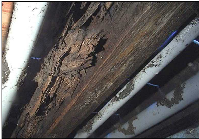
Figure 44 – Damaged Framing Near Dock C and Main Dock Connection
