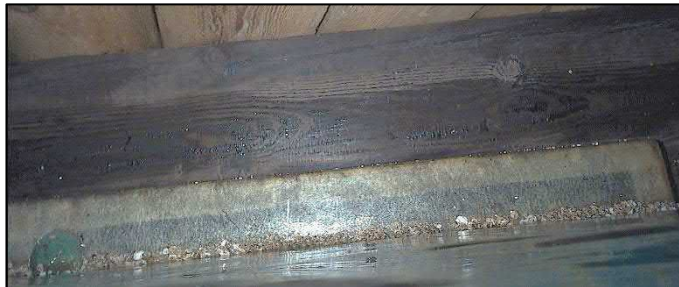
Figure 66 - Fuel Dock - Underside View with PVC Billet
