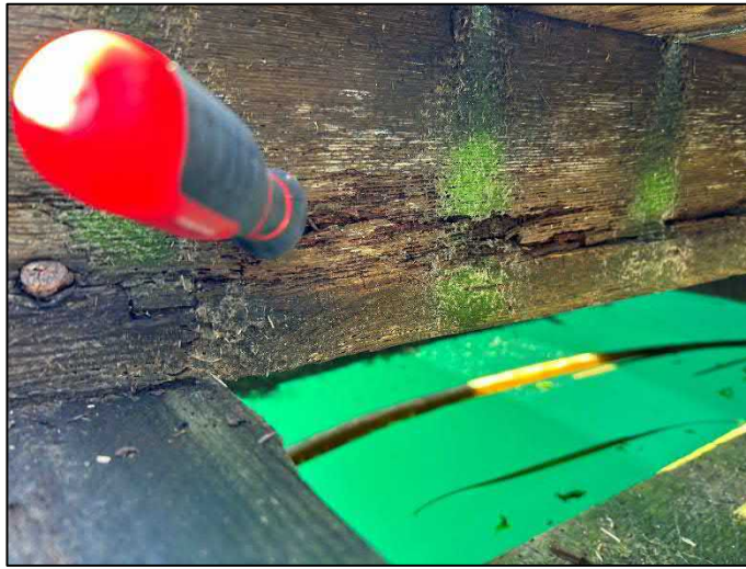
Figure 41 – Decayed Framing Near Slip B12 on Dock B
