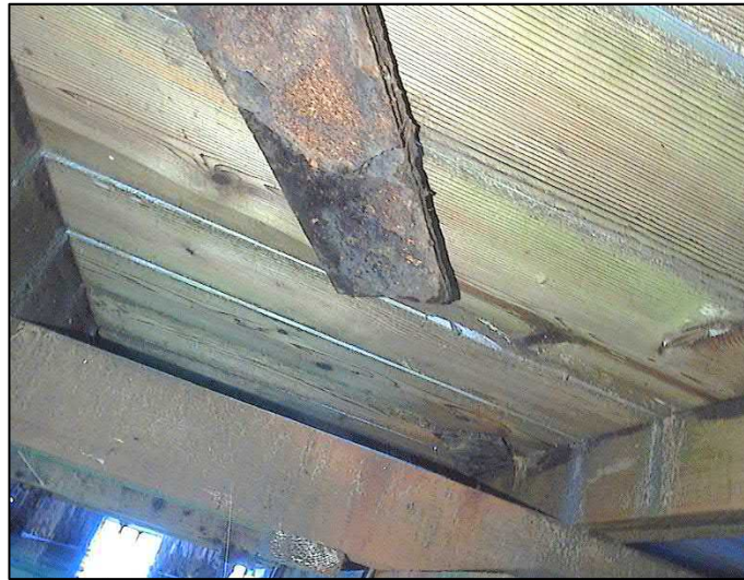
Figure 56 - Example of a Corroded and Failed Steel Brace Near T-Sections at Dock G to Dock K
