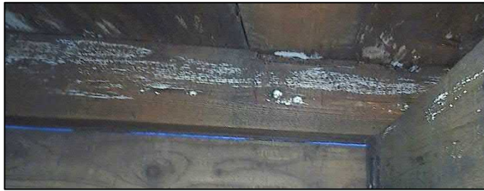
Figure 48 - Example of Fungal Growth on Framing
