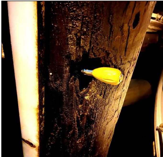
Figure 61 - Typical Hole in Timber Pile
