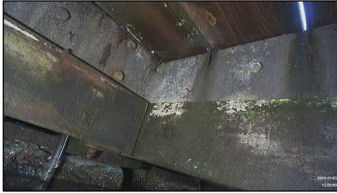
Figure 53 - Example of a Presumably Galvanized Steel Connection Plate in Good Condition
