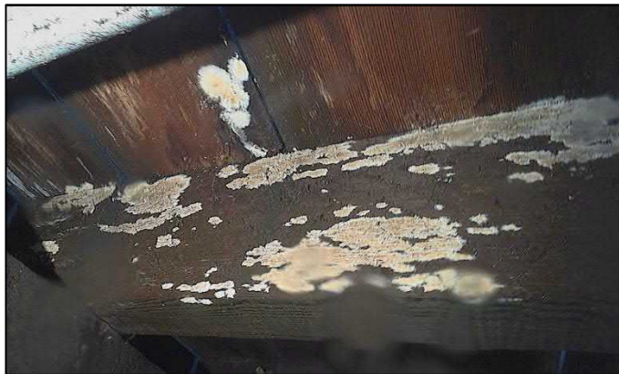
Figure 52 - Example of Fungal Growth on Framing
