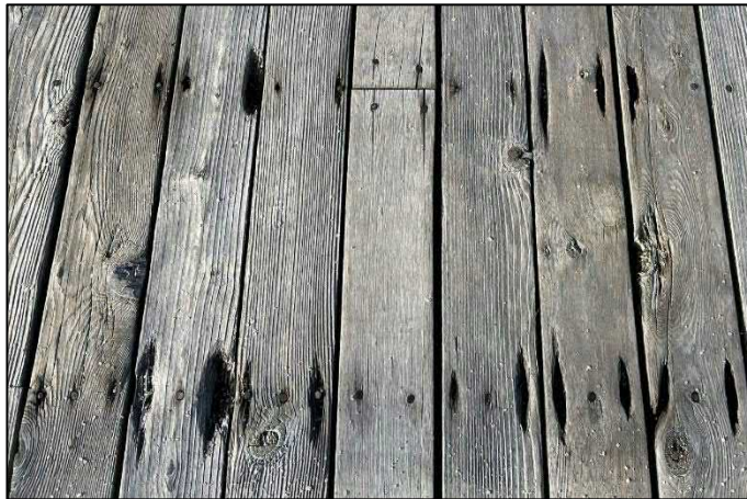
Figure 33 - Example of Deck Board Decay
