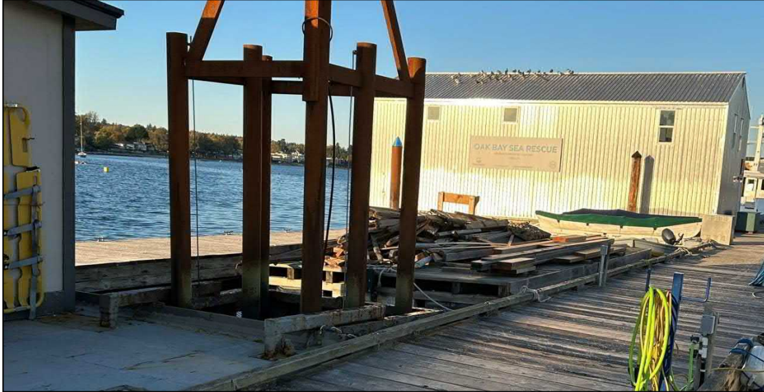
Figure 24 - Northwest Corner of Dock - Near Fuel Dock and Oak Bay Sea Rescue Facility
