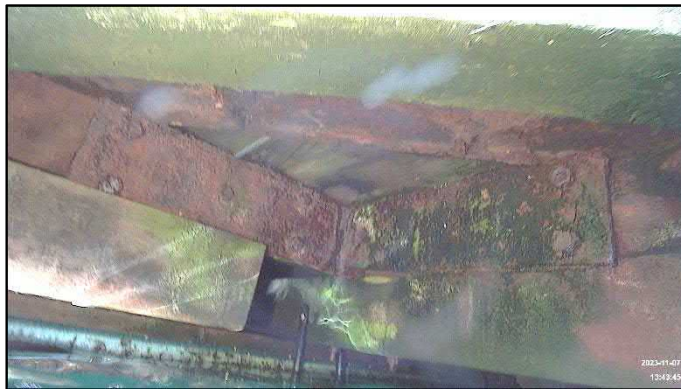
Figure 54 - Example of a Corroded Connection Plate Between Wing Dock and Main Dock
