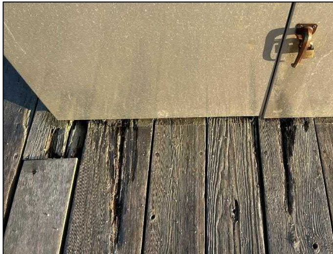
Figure 29 - Example of Deck Board Decay Near Electrical Kiosk
