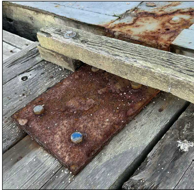
Figure 67 - Corroded Steel Plates at Fuel Dock
