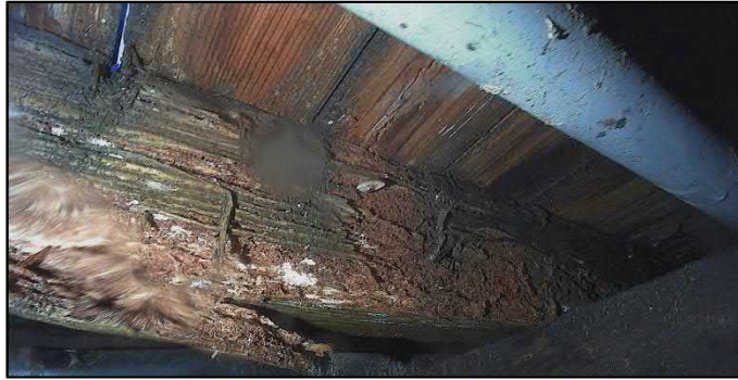
Figure 45 - Decayed Framing Near Slip E31 on Dock E
