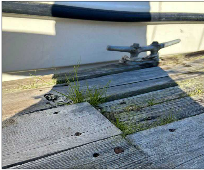
Figure 32 - Example of Deck Board Decay
