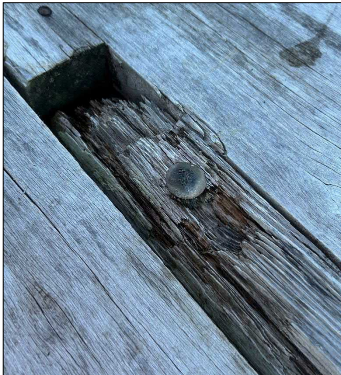
Figure 38 - Example of Decayed Connection Member at Finger Connection to Wing Dock
