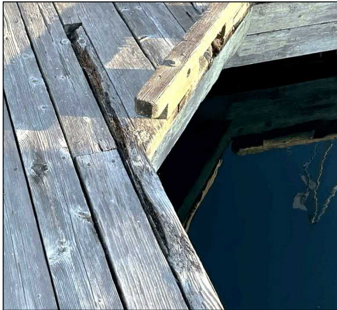
Figure 37 - Example of Decayed Connection Member at Finger Connection to Wing Dock
