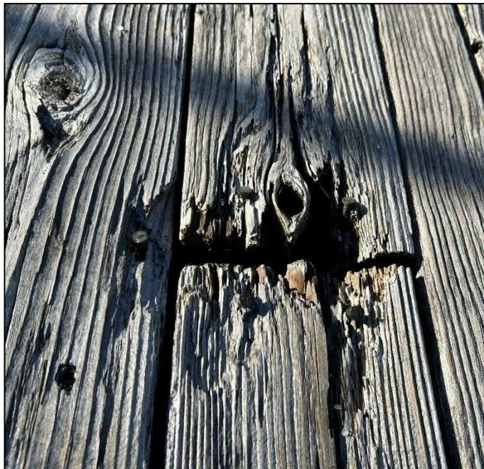
Figure 31 - Example of Deck Board Decay
