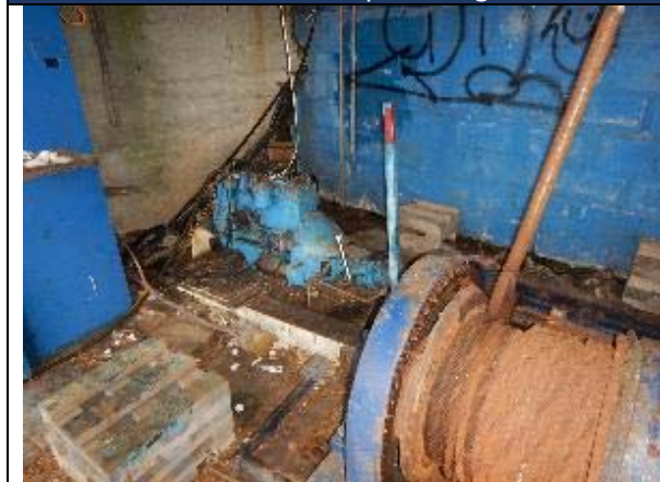
Photo 3 Description: Marine way winch system at south west extent of site
