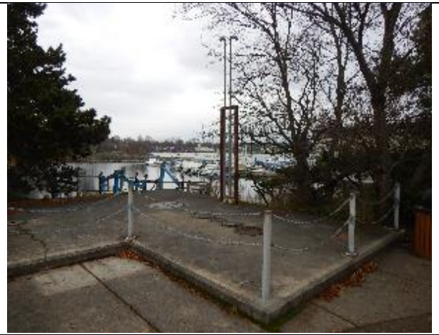
Photo 2 Description: Floating fuel dock UST area with fill caps and vent stacks at south west corner of site
