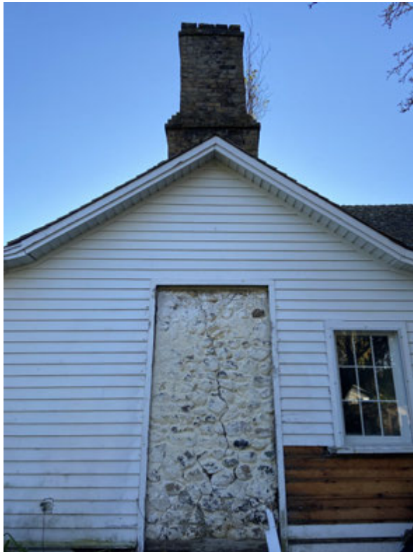
North Elevation rubble and brick chimney detail belonging to oldest part of the house.
