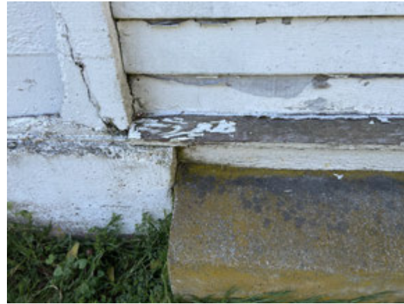
East Elevation. Different phases of concrete work built up against wall at chimney .
