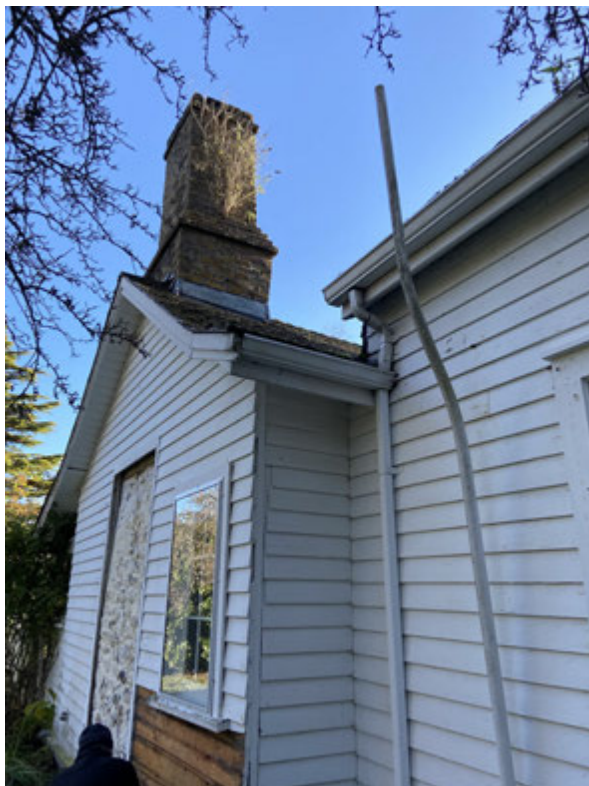
North Elevation rubble and brick chimney with connection to the 1890s addition on the right side of photo .
