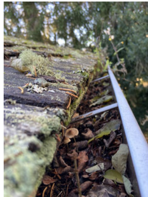
Gutters require regular cleaning.
