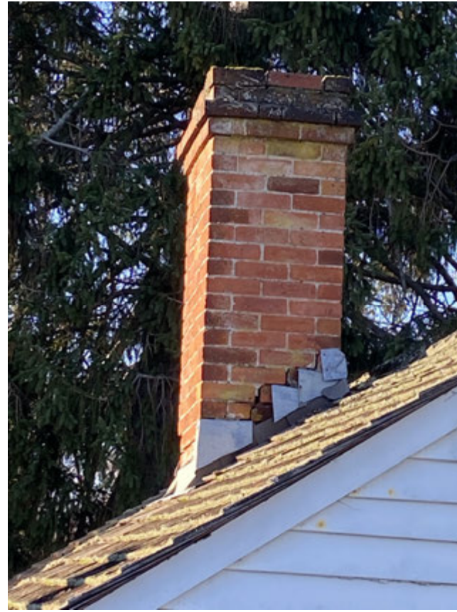
Red brick chimney over 1890s addition. Step flashings should be replaced and mortar joints re-pointed
