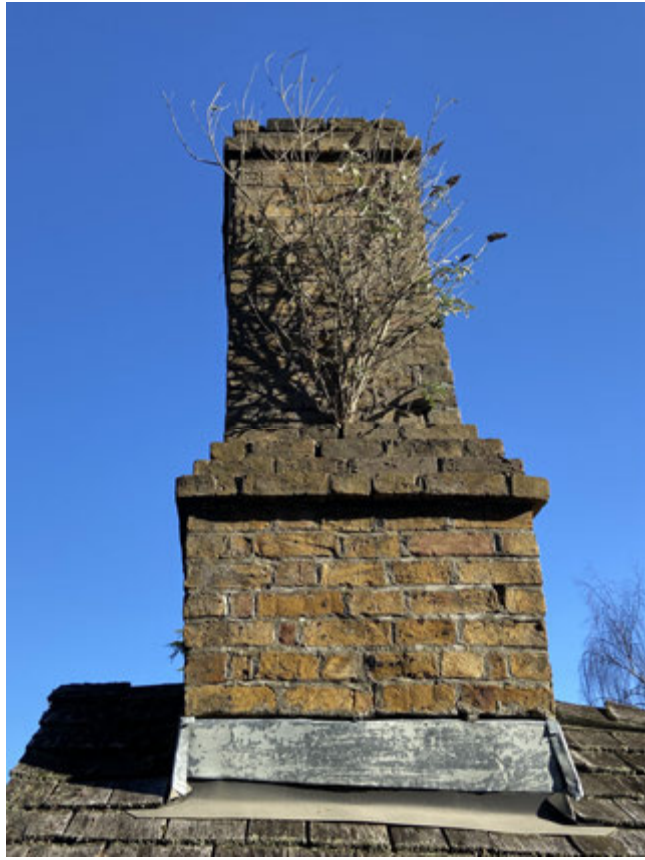
London Stock brick chimney. London bricks are a distinctive yellow/ buff colour and were imported to the new colony in the early years .
