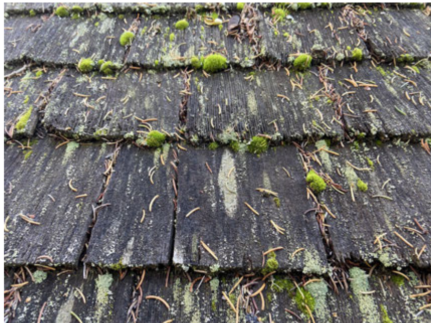
Typical condition of cedar shingles showing moss and lichen growth and debris from fir adjacent conifers..
