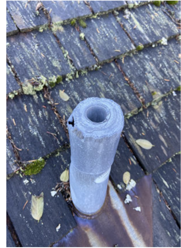
Lead flashing cover on plumbing vent pipe.
