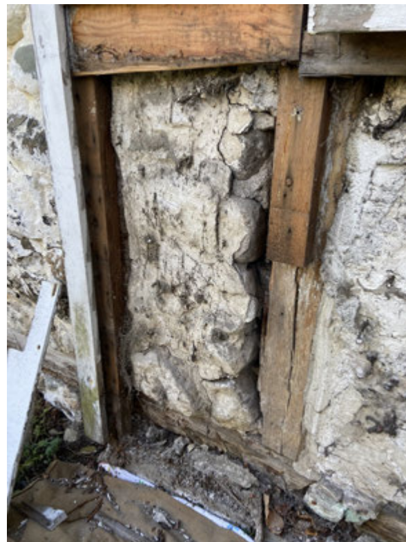
Rubble and lime mortar infill between hewn studs belonging to timber frame.
