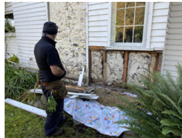
North Elevation outside kitchen. Timber framing exposed in the oldest part of the house.
