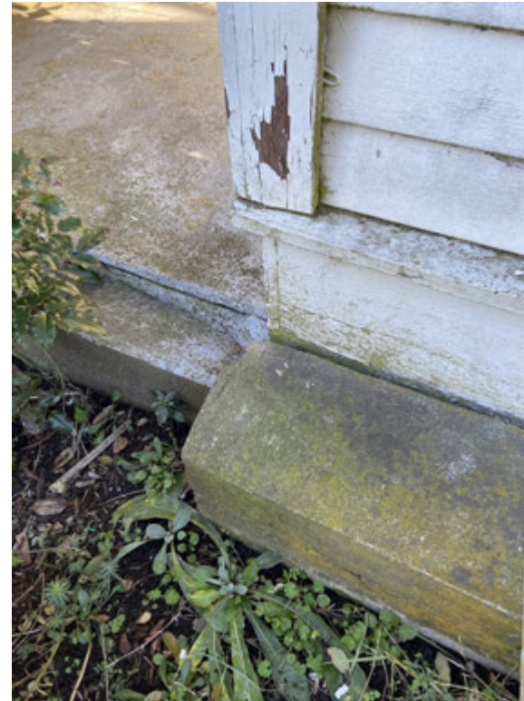
East Elevation. Gap behind curb is a vulnerable location for collecting rain and surface water.
