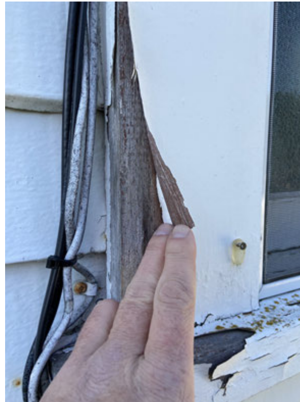
Peeling vinyl base paint (typ.) over old red ochre paint on window trims.
