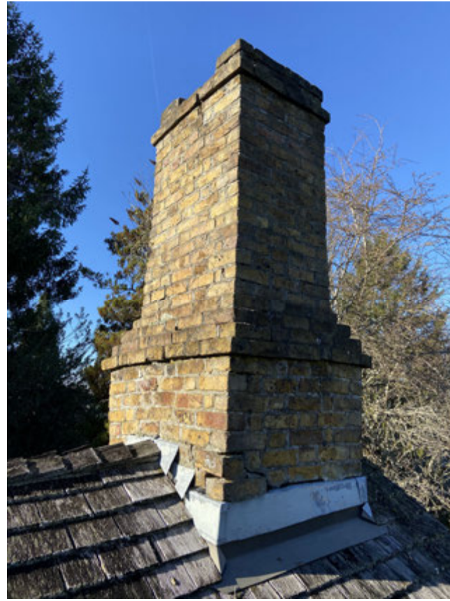
Chimney flashings require replacing and the lower brick courses repointing. Vegetation should be removed and joints repointed mortar is missing or detached.
