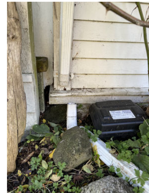
Northeast corner. Detached downspout and surface drain typical of most downspouts.
