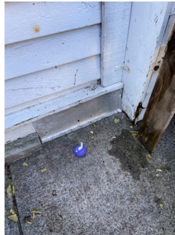
East Elevation. Rear patio rodent proofing at foundation level.
