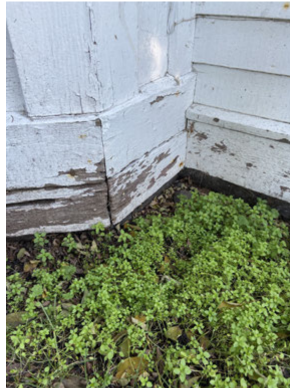
West Elevation, bay window. Heavily weathered trim boards at foundation level.
