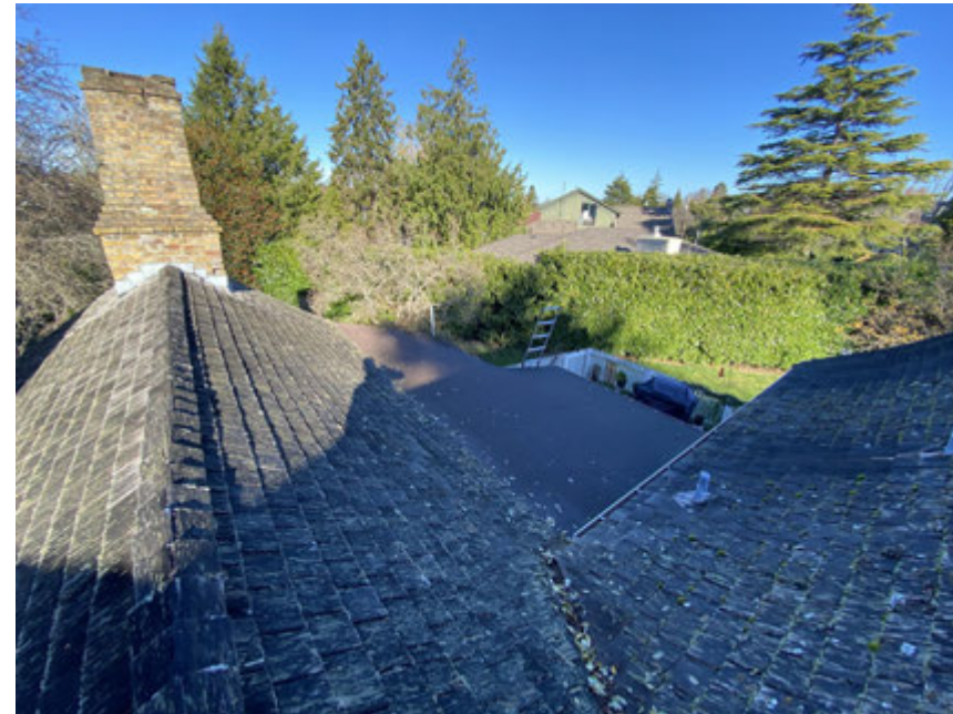
Roof and chimney over 1850s range. Asphalt roof over kitchen extension. Photo facing northeast.
