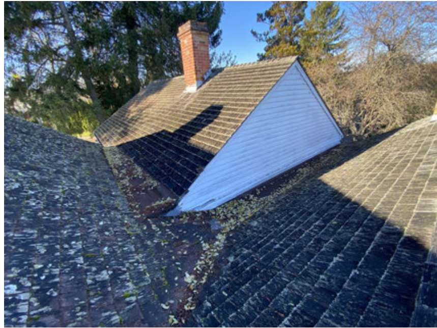
Roof over 1890s addition facing northwest. Valley gutters are full of leaf litter.
