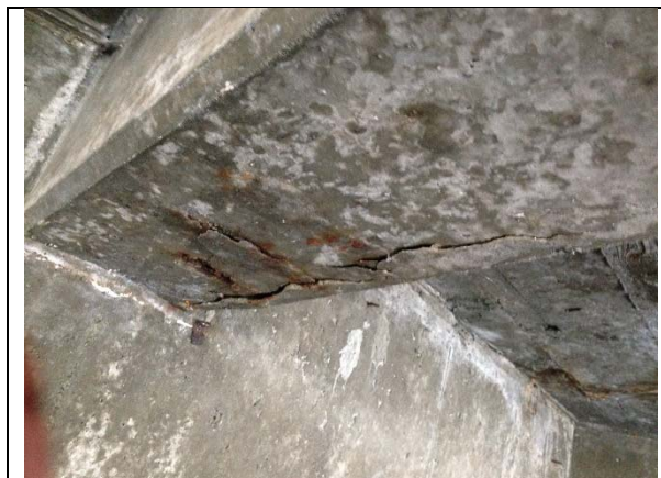
Figure 25-D: Sample of spalling concrete.
