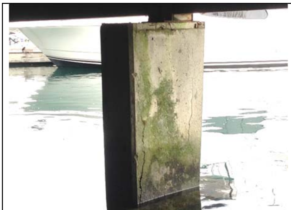
Figure 25-C: Cracks and saltwater ingress at column supporting restaurant has reduced strength and accelerated corrosion.
