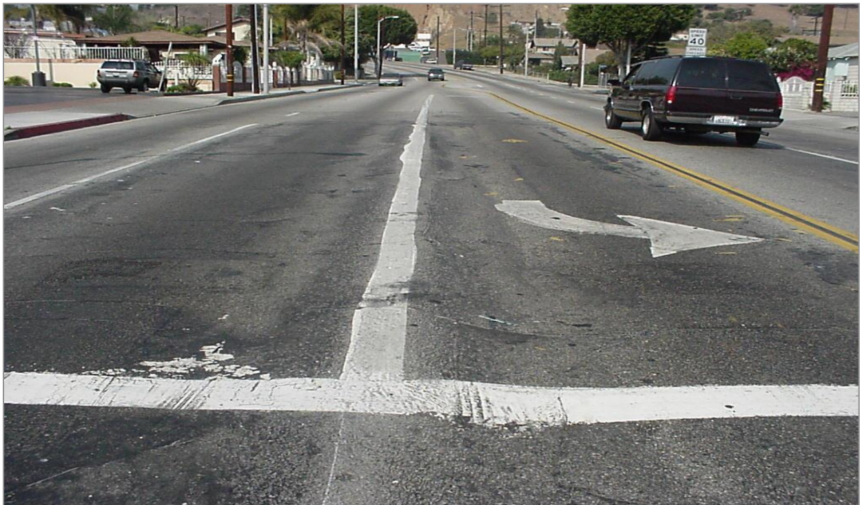
Figure 4.25: Severe Wheel Track Rutting (Image used for illustration)
