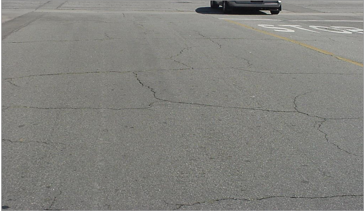
Figure 4.12: Moderate Block/Map Cracking (Image used for illustration)
