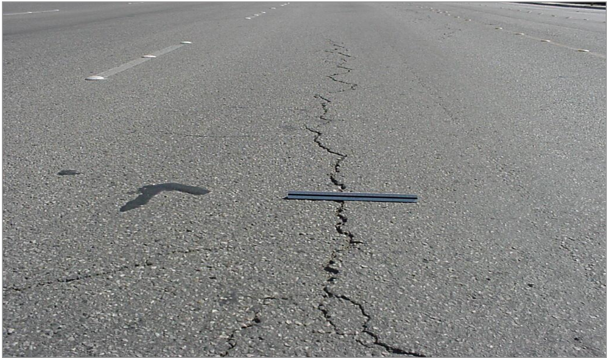
Figure 4.17: Severe Longitudinal Cracking (Image used for illustration)
