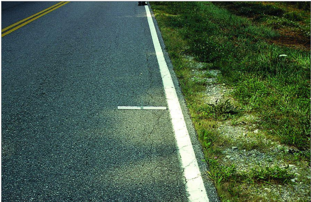
Figure 4.6: Slight Edge Cracking (Image used for illustration)
