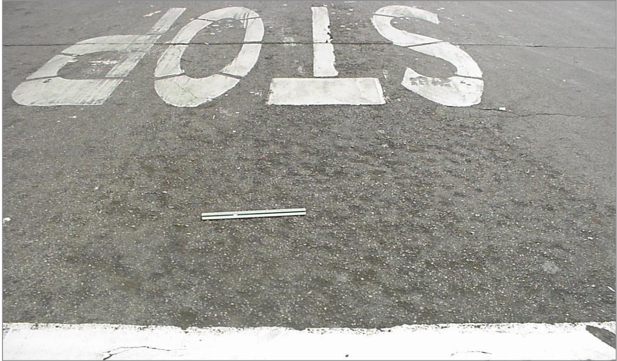
Figure 4.45: Severe Raveling (Image used for illustration)
