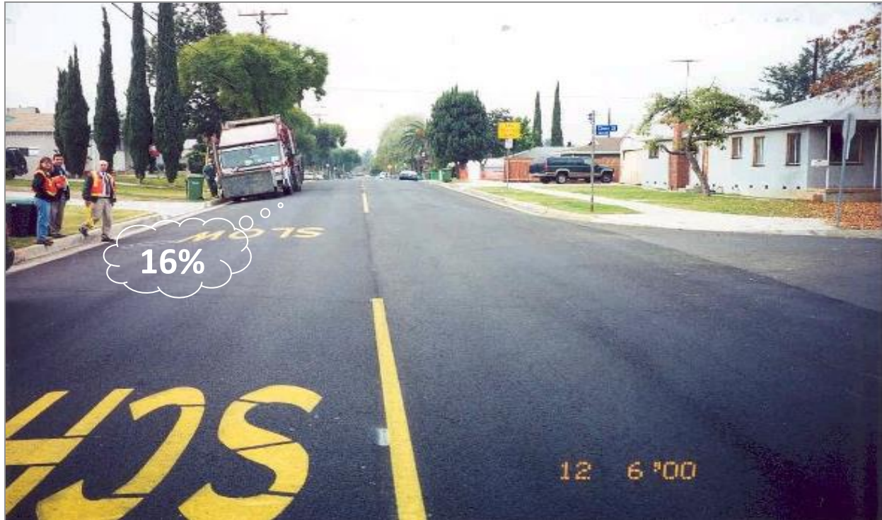
Figure 4.37: Severe Excessive Crown (Image used for illustration)
