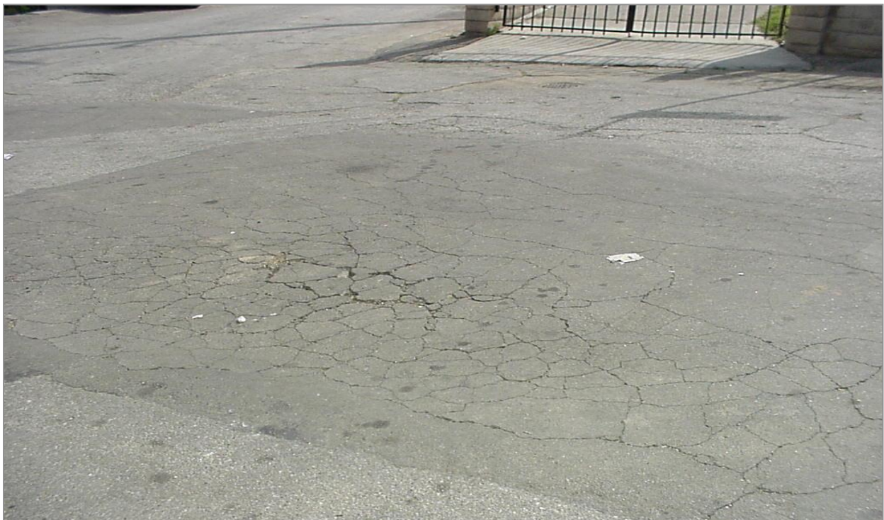
Figure 4.53: Severe (Failed) Patch (Image used for illustration)
