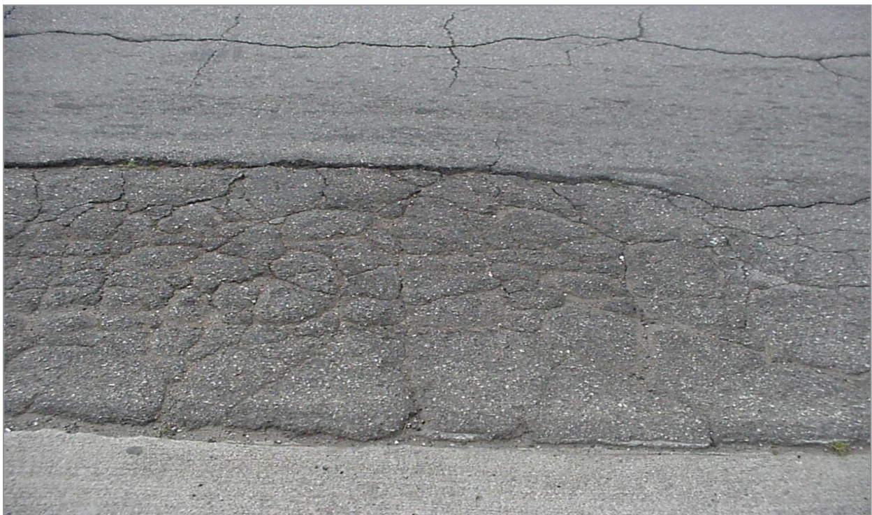
Figure 4.8: Severe Edge Cracking (Image used for illustration)
