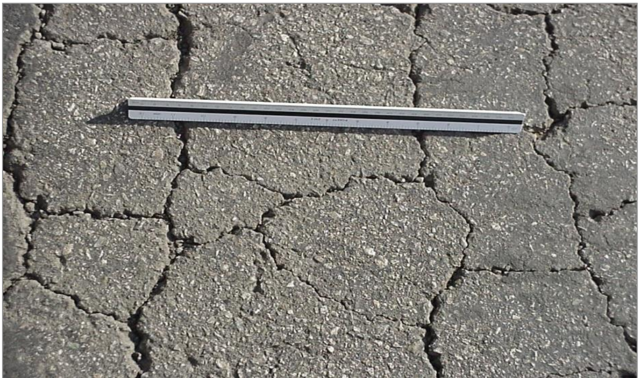
Figure 4.3: Moderate Alligator Cracking (Image used for illustration)
