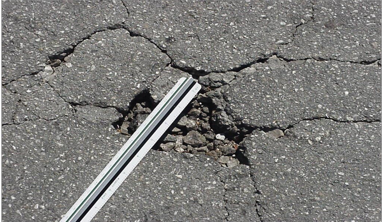
Figure 4.39: Slight Pothole (Image used for illustration)
