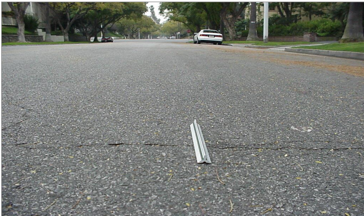
Figure 4.19: Moderate Transverse Crack (with random cracking) (Image used for illustration)
