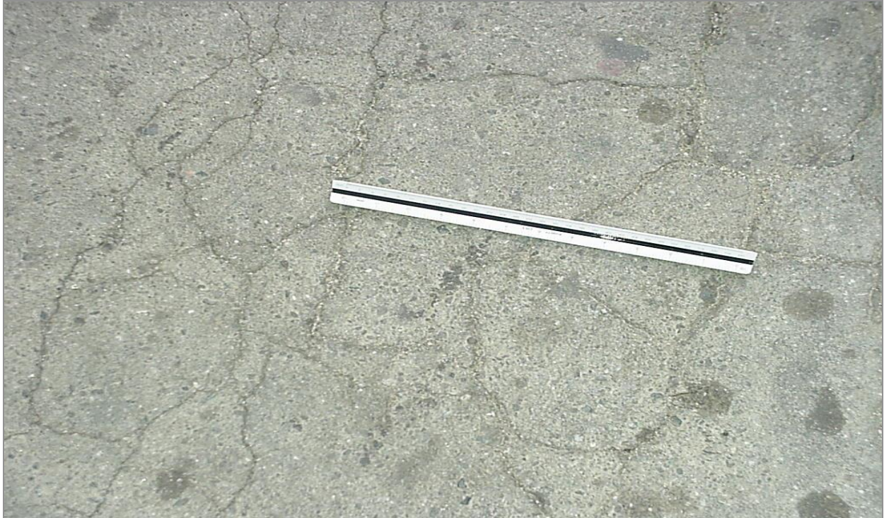
Figure 4.2: Slight Alligator Cracking (Image used for illustration)
