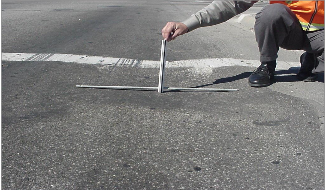
Figure 4.24: Moderate Wheel Track Rutting (Image used for illustration)
