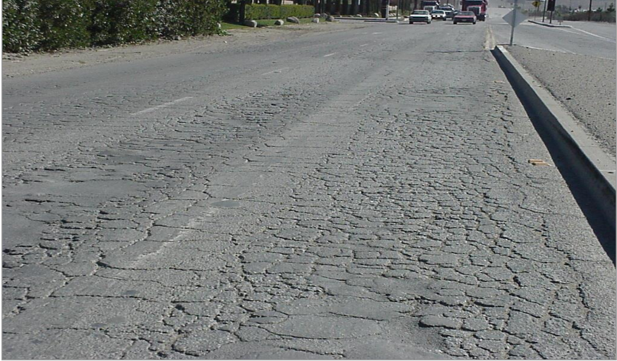
Figure 4.4: Severe Fatigue (Alligator) Cracking (Image used for illustration)
