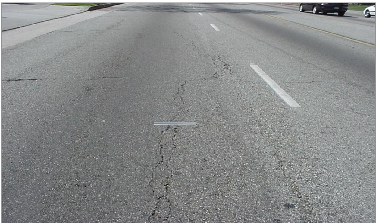
Figure 4.16: Moderate Longitudinal Cracking (Occurs in Wheel Path – rated as Fatigue Cracking) (Image used for illustration)
