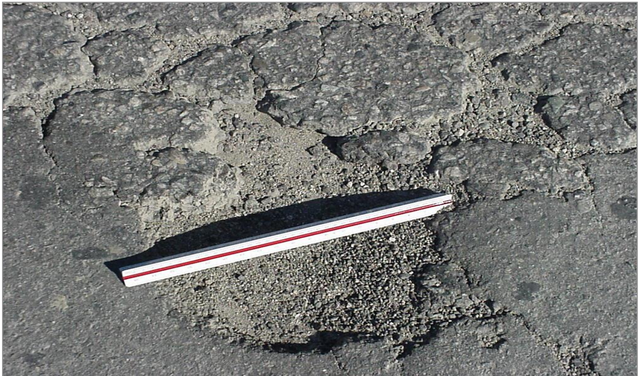
Figure 4.41: Severe Pothole (Image used for illustration)
