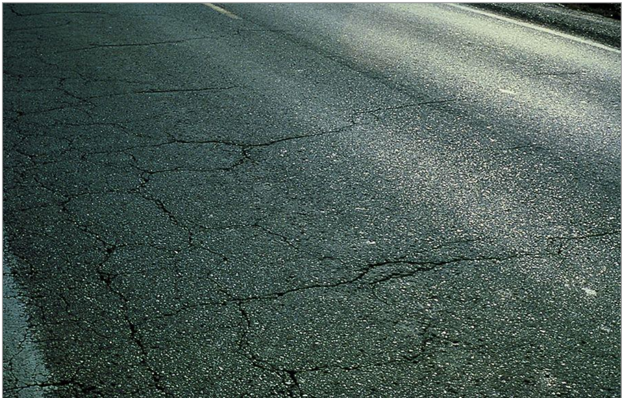
Figure 4.13: Block/Map Cracking (Image used for illustration)
