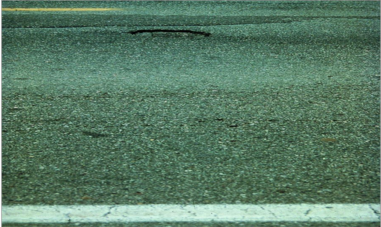
Figure 4.40: Moderate Pothole (Image used for illustration)
