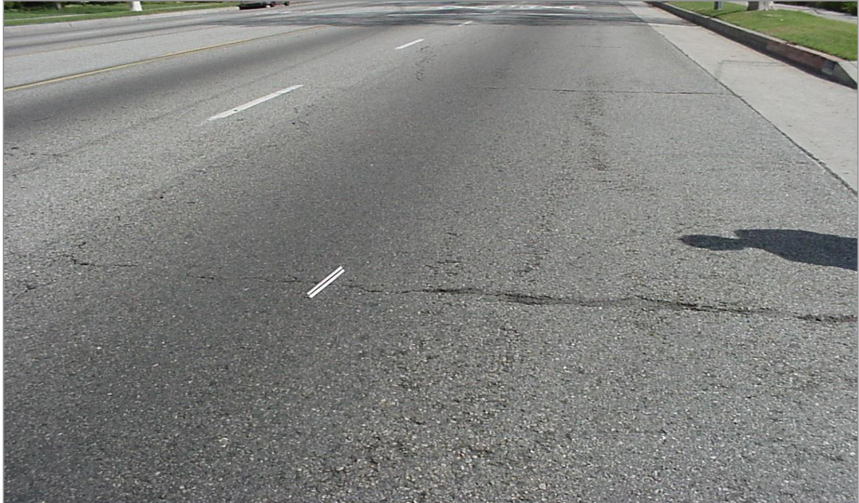
Figure 4.20: Moderate Transverse Crack (Image used for illustration)
