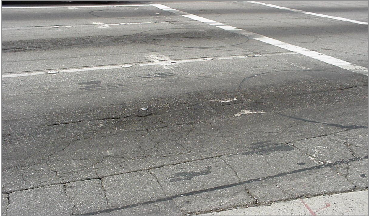
Figure 4.7: Moderate Edge Cracking (Image used for illustration)
