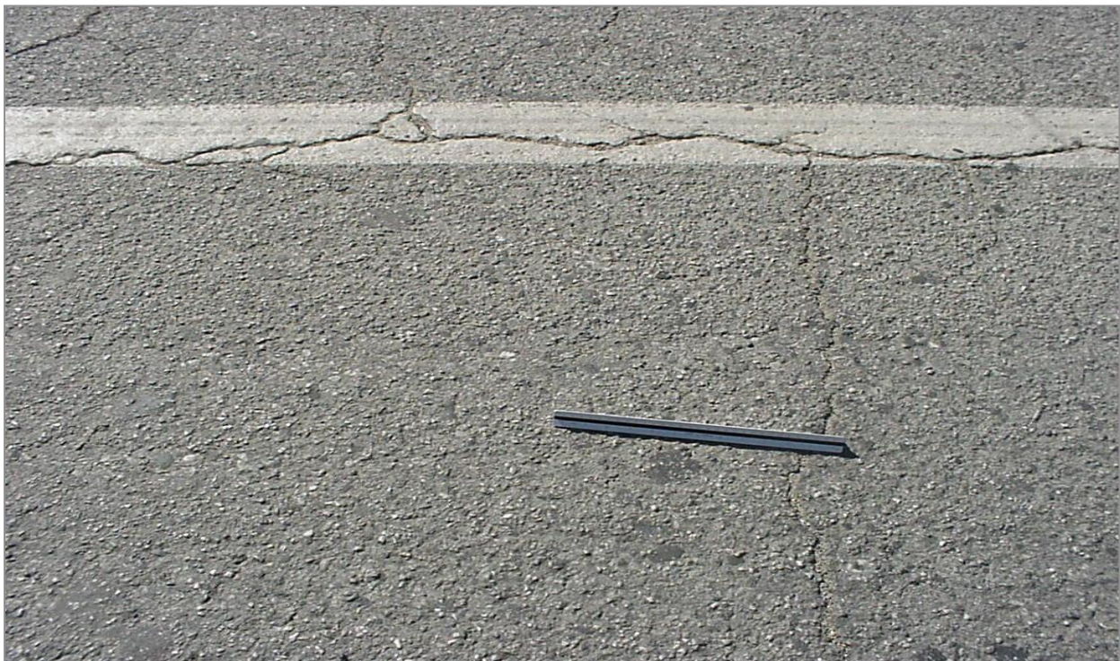
Figure 4.11: Slight Block/Map Cracking (Image used for illustration)
