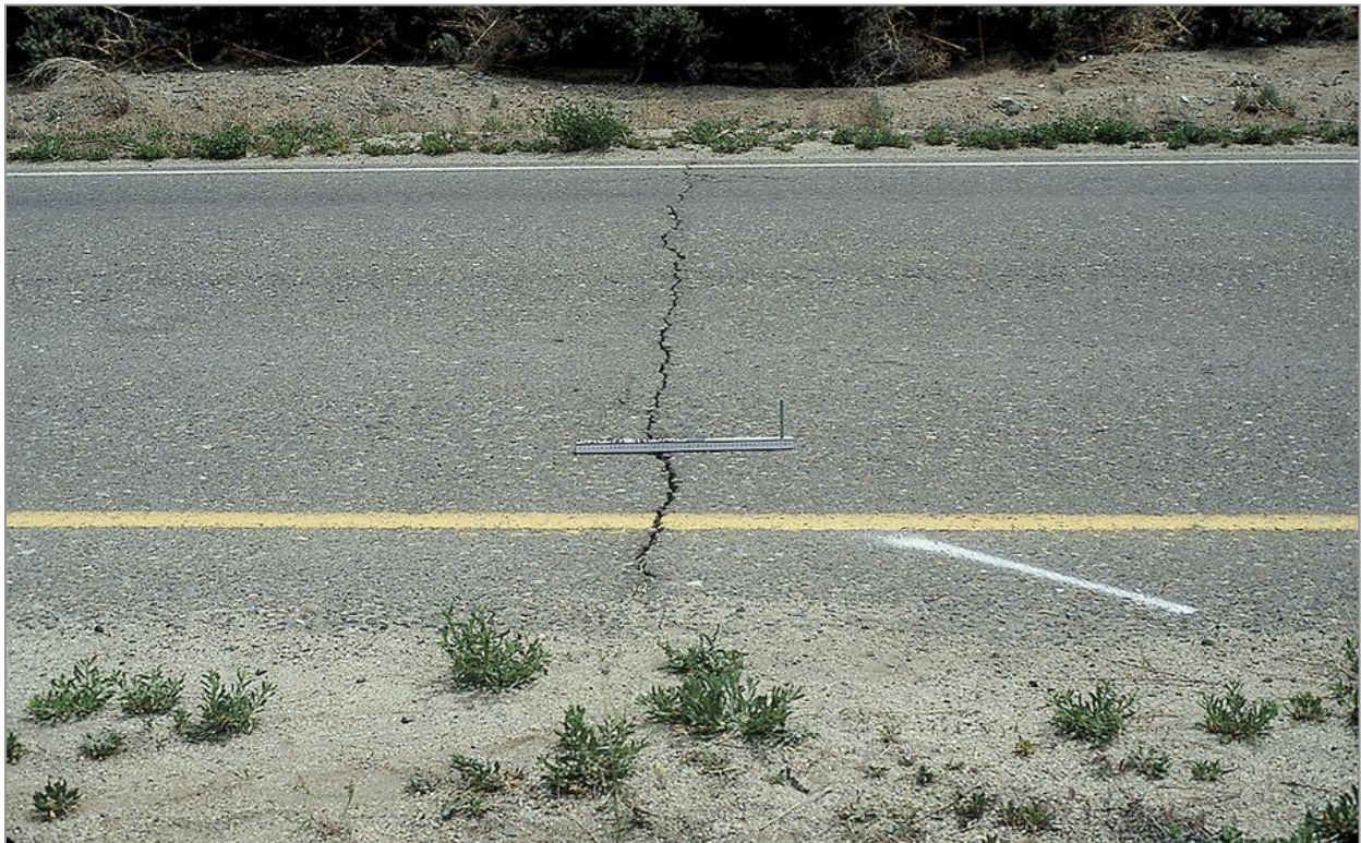
Figure 4.21: Severe Transverse Crack (Image used for illustration)
