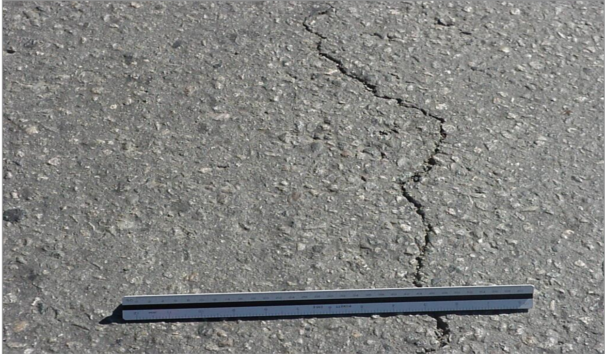
Figure 4.15: Moderate Longitudinal Cracking (Image used for illustration)
