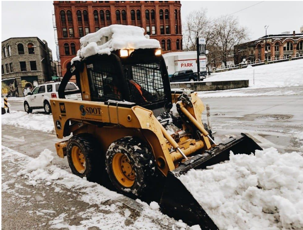
Example of snow clearing in a protected bike lane. Image credit: Seattle Department of Transportation
