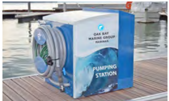
Marine Sewage Pump Out
