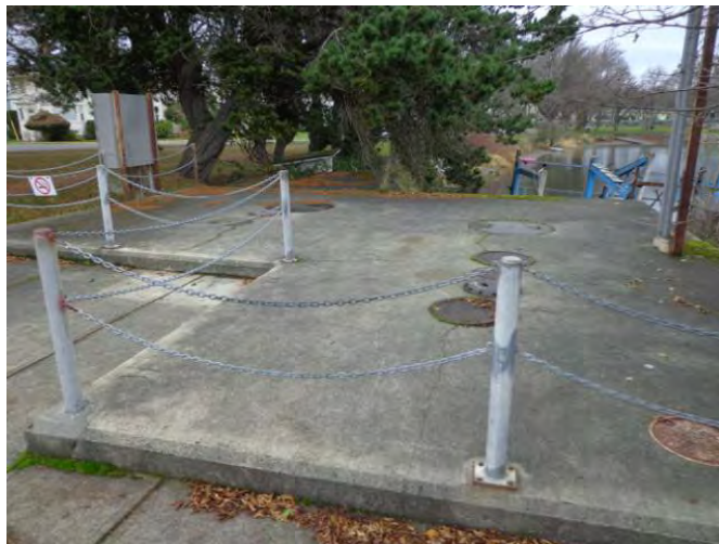
Photo #51: In-ground Gas and Diesel Pumps
