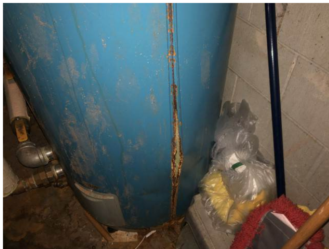
Photo #24: Restaurant Hot Water Tank Bulging.
