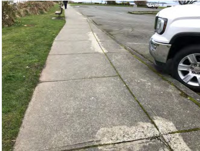
Photo #64: Concrete Sidewalk Settlement.
