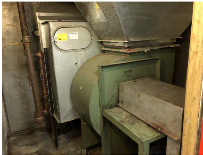
Photo #17: Restaurant Air Handling Unit.
