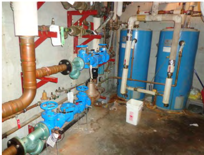
Photo #23: Incoming Water Line and Restaurant Branch Lines and Hot Water Storage Tanks
