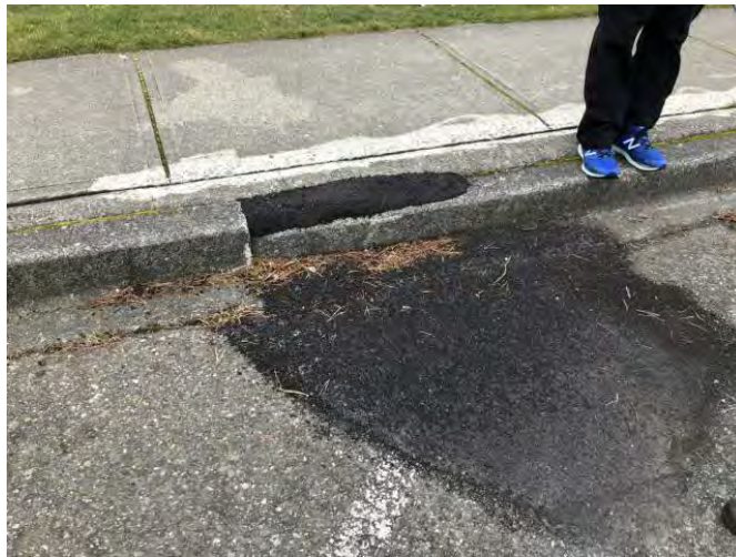
Photo #62: Parking Lot Asphalt Patch.
