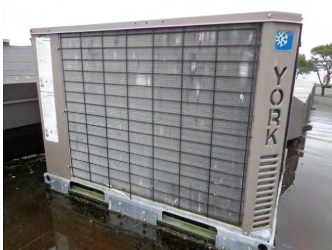
Photo #19: Restaurant Condensing Unit
