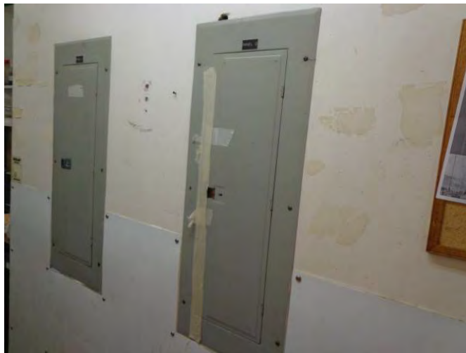
Photo #27: Restaurant Electrical Distribution Panels
