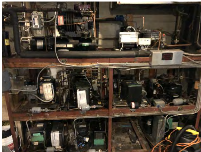
Photo #21: Restaurant Refrigeration Compressors.
