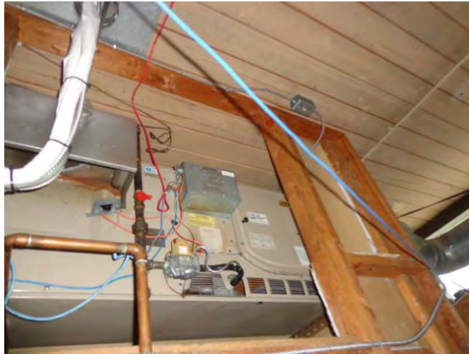
Photo #34: Office In-ceiling Gas-fired Furnace
