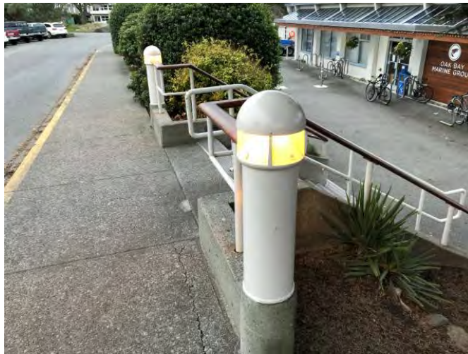
Photo #74: Site Bollard Lights - Typical.
