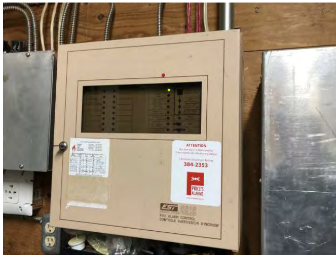
Photo #71: Main Fire Alarm Panel.
