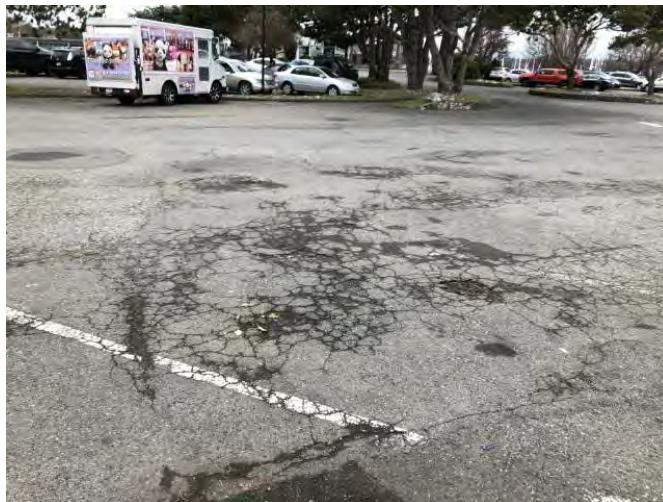
Photo #63: Parking Lot Cracking - Typical.
