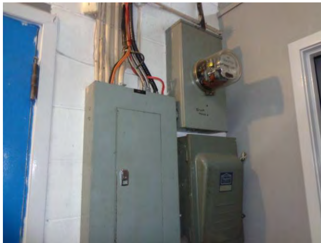
Photo #45: Dockworks Electrical Distribution Panel
