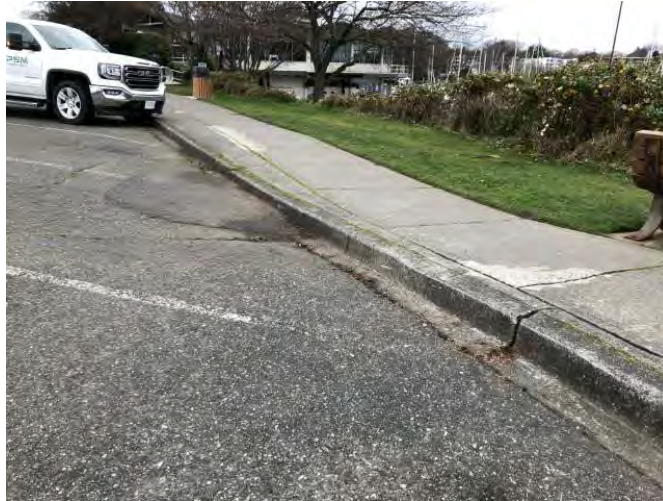
Photo #61: Parking Lot Settlement.
