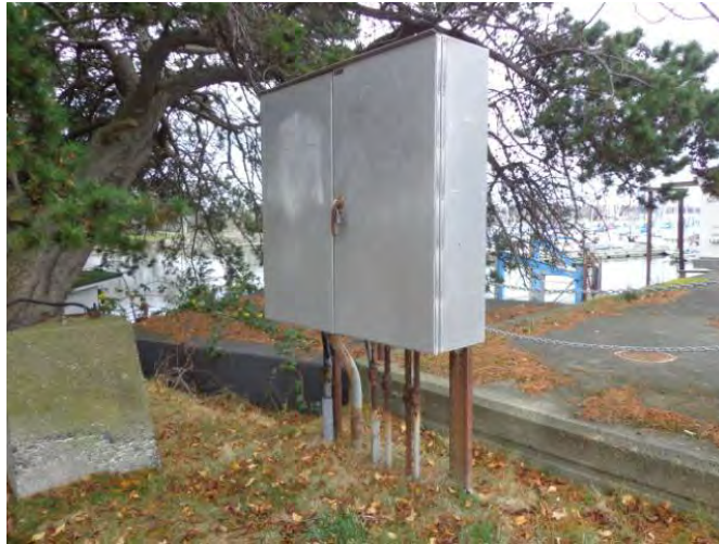
Photo #52: Gas and Diesel Pump Controllers
