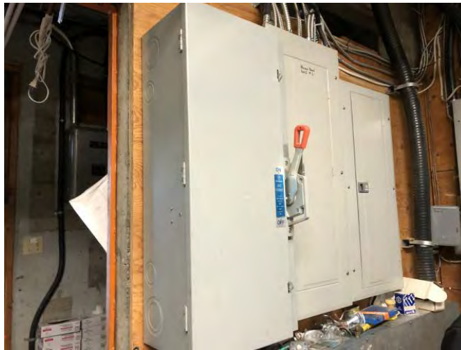
Photo #73: Main Electrical Distribution Panels.
