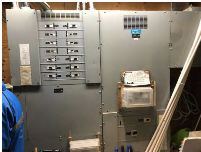
Photo #72: Main Electrical Switchgear.
