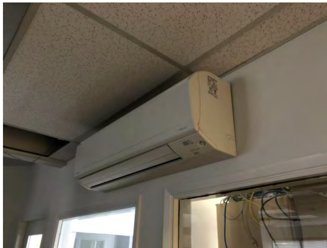
Photo #35: Office Split-System Air Conditioning Unit.
