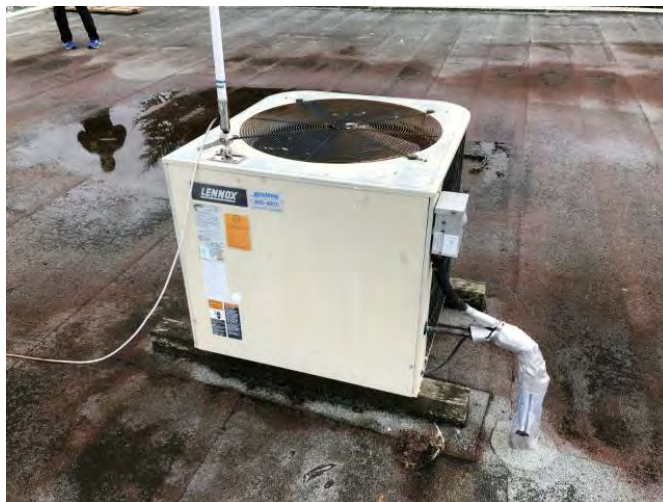
Photo #36: Office Condensing Unit - Typical.
