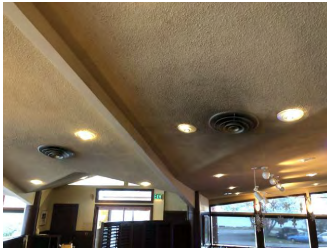
Photo #20: Restaurant Ceiling Diffusers - Typical.
