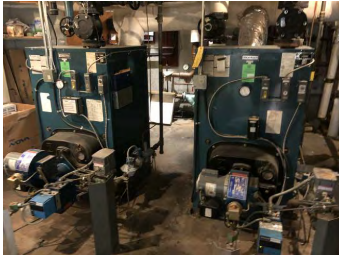
Photo #22: Restaurant Gas-fired Boilers.
