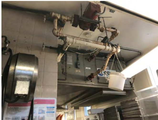
Photo #18: Restaurant Make-up Air Unit.
