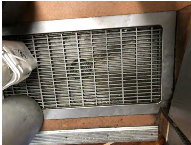
Photo #25: Restaurant Kitchen Trench Drain.
